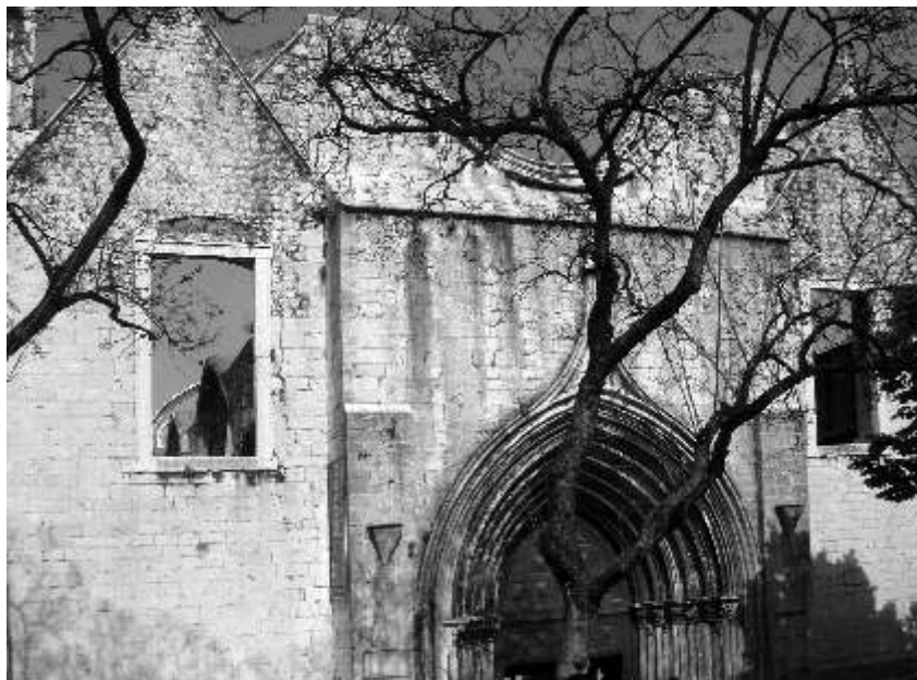
An old church with only the outside walls still left from the Lisbon earthquake
